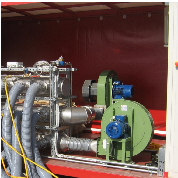
1. FORCED VENTILATION SYSTEM
